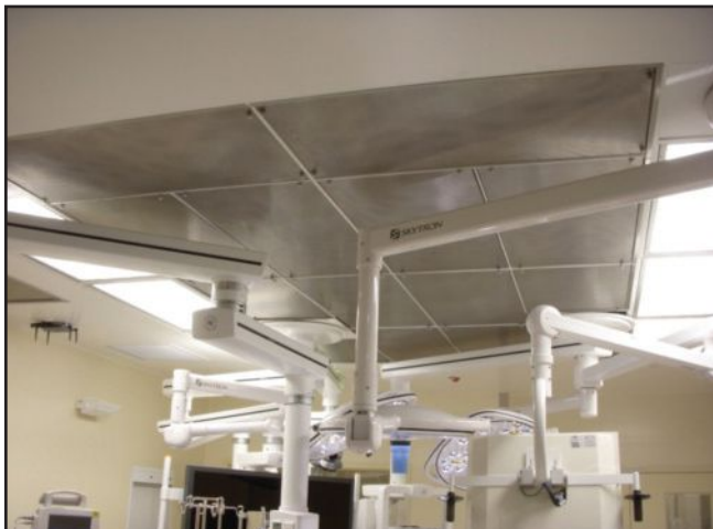
FIGURE 2. Finished OR suite with 40% open S/S perforated grilles on downstream side.
