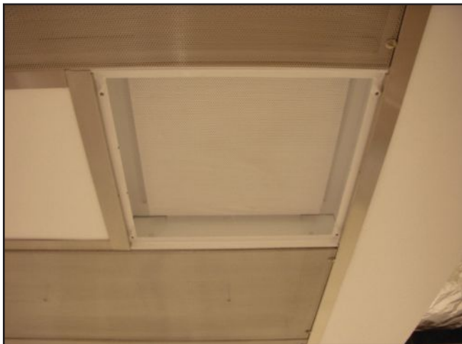
FIGURE 1. Typical view inside laminar flow modules (post perforated basket installation).
